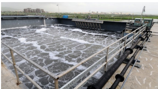
Figure 22.4 A view of sewage treatment plant
